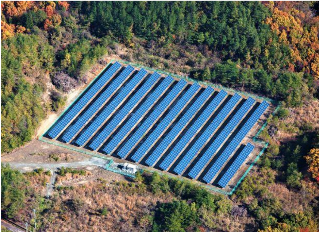
Figure 6: CS Koriyama-shi Power Plant (Fukushima Prefecture) (0.6 MW)
